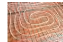
Floor heating loop
