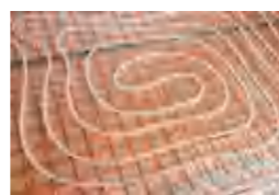
Floor heating loop
